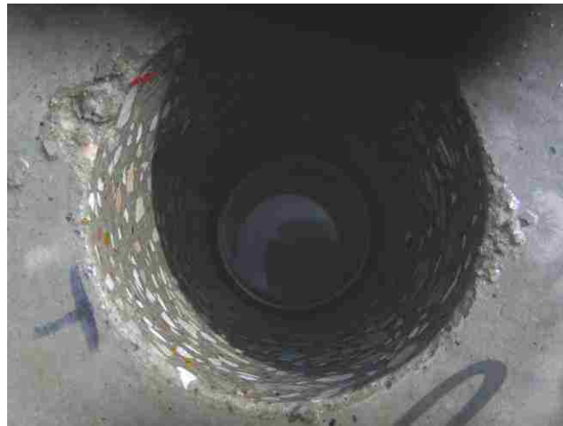
Figure 5.17 Drilled core in beam.
